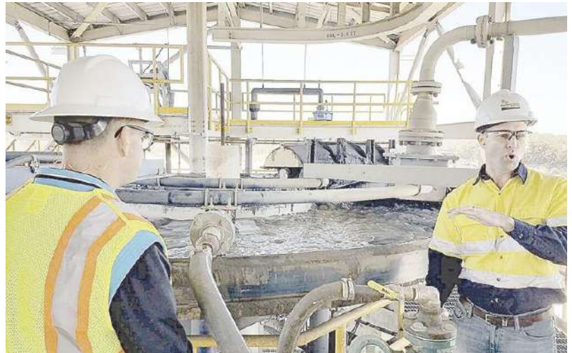
Stuart Forrester (right) explains the mineral separation process at Chemours (Southern Ionics) sand filtration plant in Offerman. - The Blackshear Times photo
